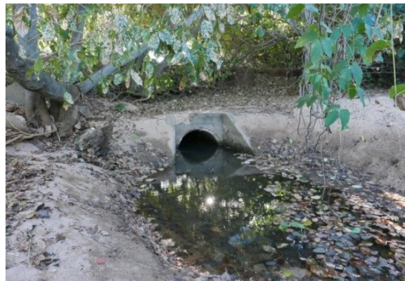
Figure 5. Progress Drive pipe outfall opposite Hickory Street, ponding water
